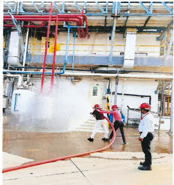
Safety Squad members operated the firefighting system to create a water curtain.
