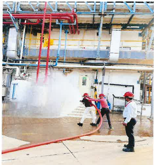
Safety Squad members operated the firefighting system to create a water curtain.
